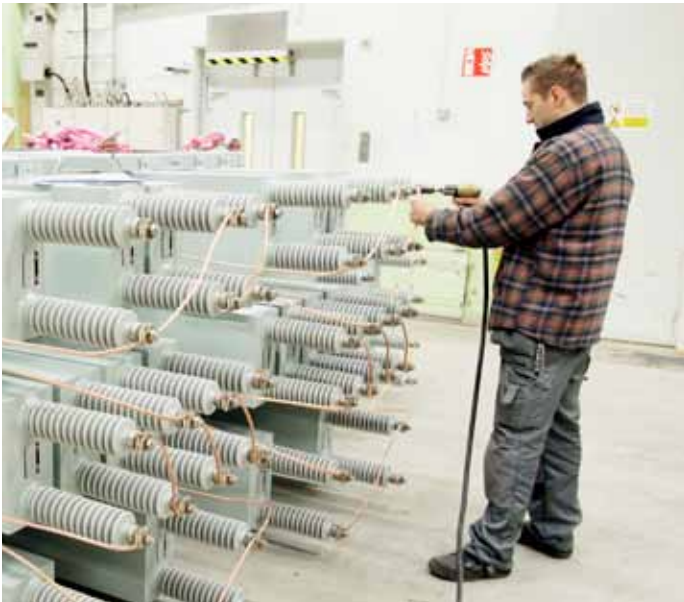
Internal wiring, connection of bushings
